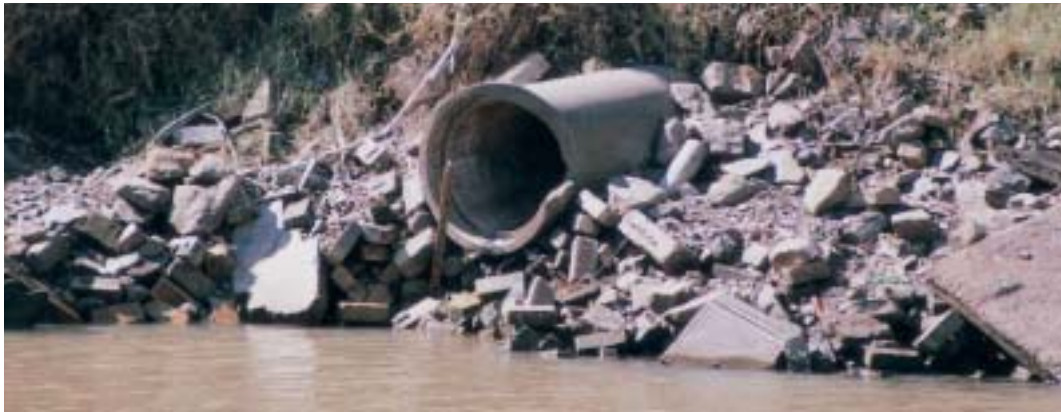
Stormwater pipe carrying stormwater runoff directly into the river and reducing water quality. Photo Guy Roth.
