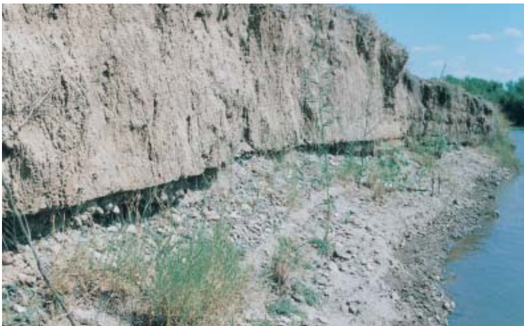
A riverbank with no riparian vegetation to protect it from erosion. Photo Guy Roth.
