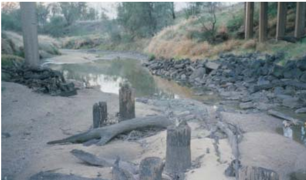
Rock riprap is being used on this part of the Condamine River to protect the toe of the bank which is gradually eroding away and threatening the bridge supports. Photo Guy Roth.
