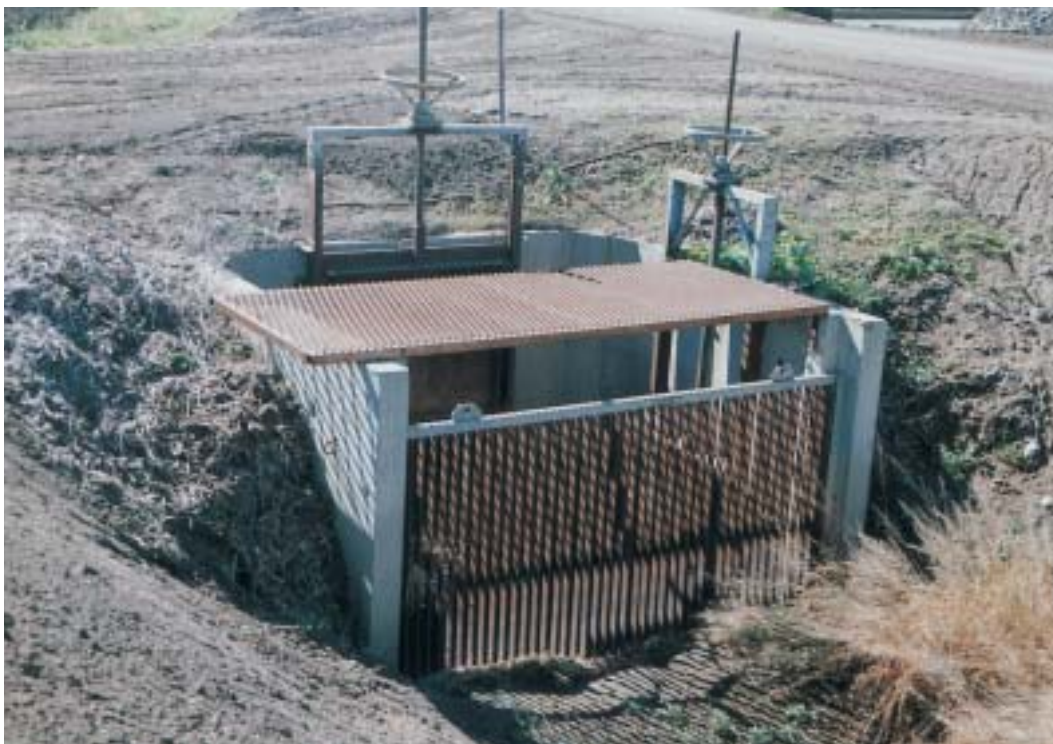
Drop box incorporated into farm irrigation system. Photo Guy Roth.
