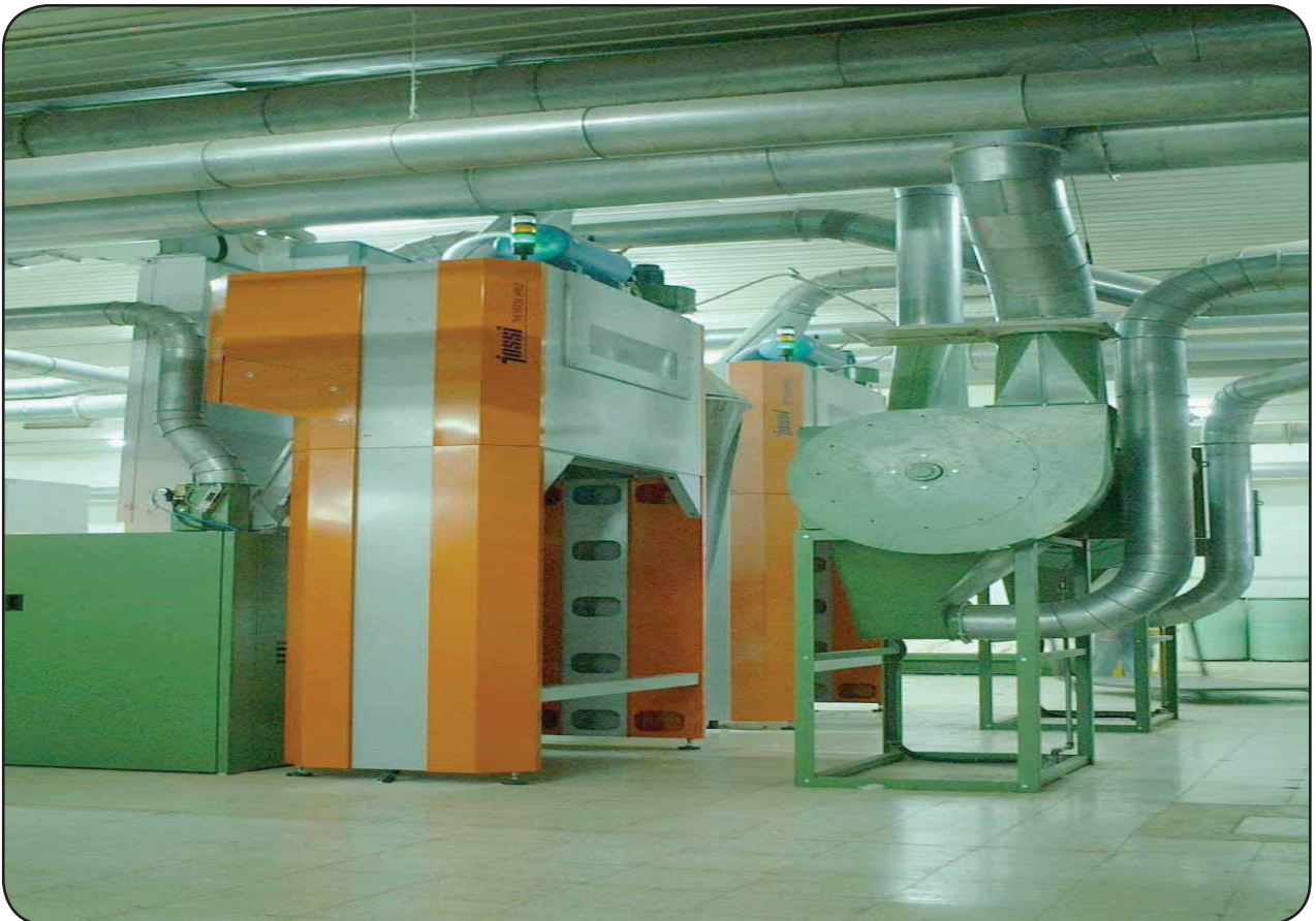
Figure 6 – Blowroom equipped with Jossi detection systems (photo courtesy of Jossi Systems AG)
