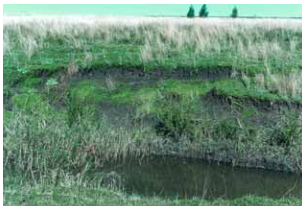
Lippia can cause severe cracking, destabilizing banks and causing slumping. (Photo: Mike Lucy)
